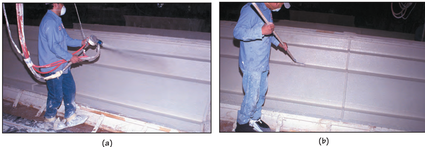
FIGURE 28.55 (a) Spraying of a GFRC mix over the mist coat. (b) Consolidating the GFRC mix using a roller around the bends, edges, and corners.
