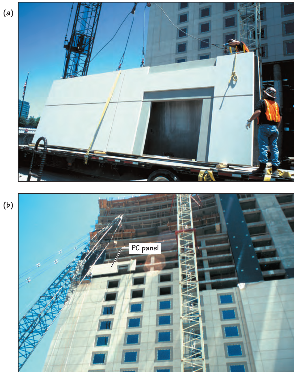
FIGURE 28.38 (a) A precast concrete panel being unloaded from the delivery truck for hoisting into position by a crane. (b) The same panel being hoisted into its final position.
