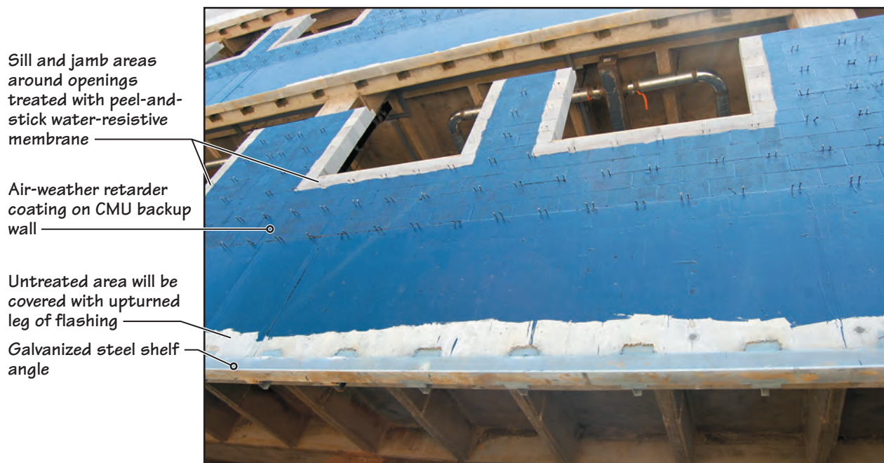
FIGURE 28.25 The exterior surface of a CMU backup wall (and the underlying spandrel beam) has been treated with a liquid air-weather retarder (blue color) before the brick veneer is constructed.
